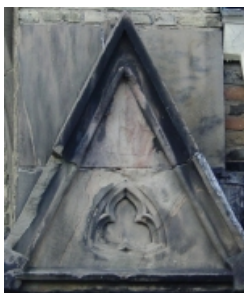
Time, weather and pollution have damaged the stone and brickwork.
